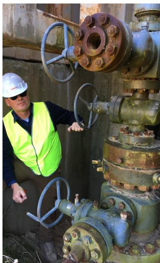
Established wellhead infrastructure at PL231 Reid's Dome.
