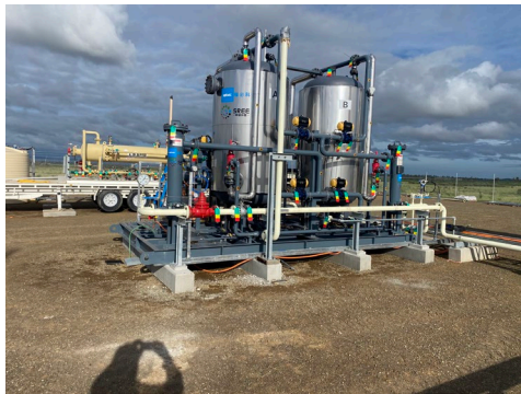
Figure 2: Low pressure gas dehydrator designed to remove moisture as it passes through two contactor desiccant vessels
