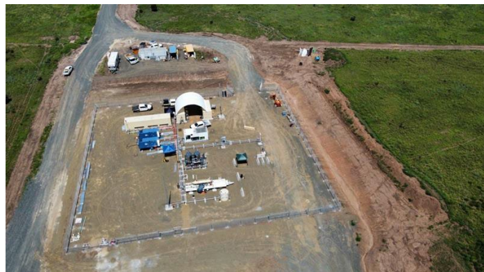
Figure 1: Near Complete CNG Facility including all weather access road (top of photo) leading to Carnarvon Highway.
