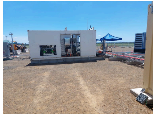
Figure 3: Refurbished Four Stage CNG Compressor capable of 25000 Kpa (3750 psi). CNG in a box
