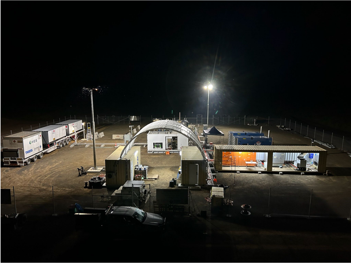
Figure 1: Completed CNG Facility with virtual pipeline trailer parked at the filling post, in preparation for commissioning
