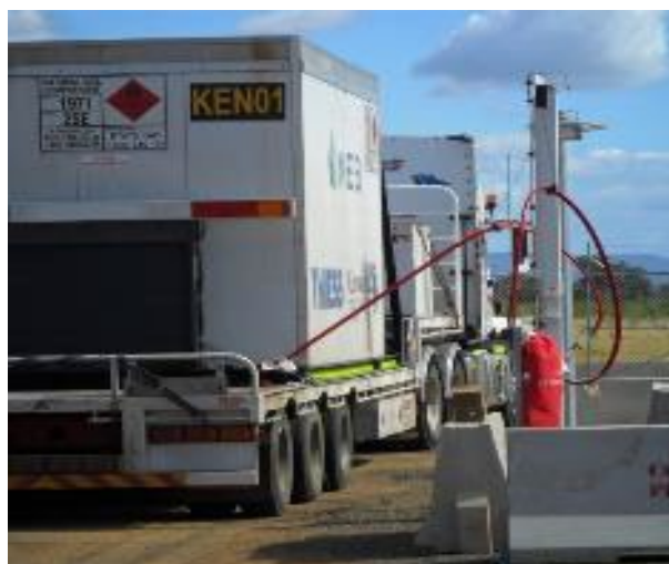
Figure 4: Loading post and filling of virtual pipeline trailers.
