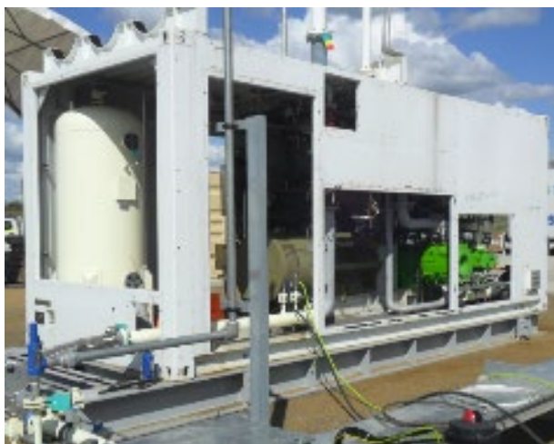
Figure 2: Commissioned modular compressor package, capable of compressing up to 1.7TJ of natural gas per day
