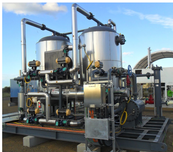
Figure 3: Commissioned dehydrator package, capable of reducing moisture content to less than 35mg/sm 3
